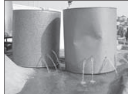
Water tanks on a Palestinian home in Hebron punctured by Israeli settlers (14 April 2009). Photo: palestinesolidarityproject.org
